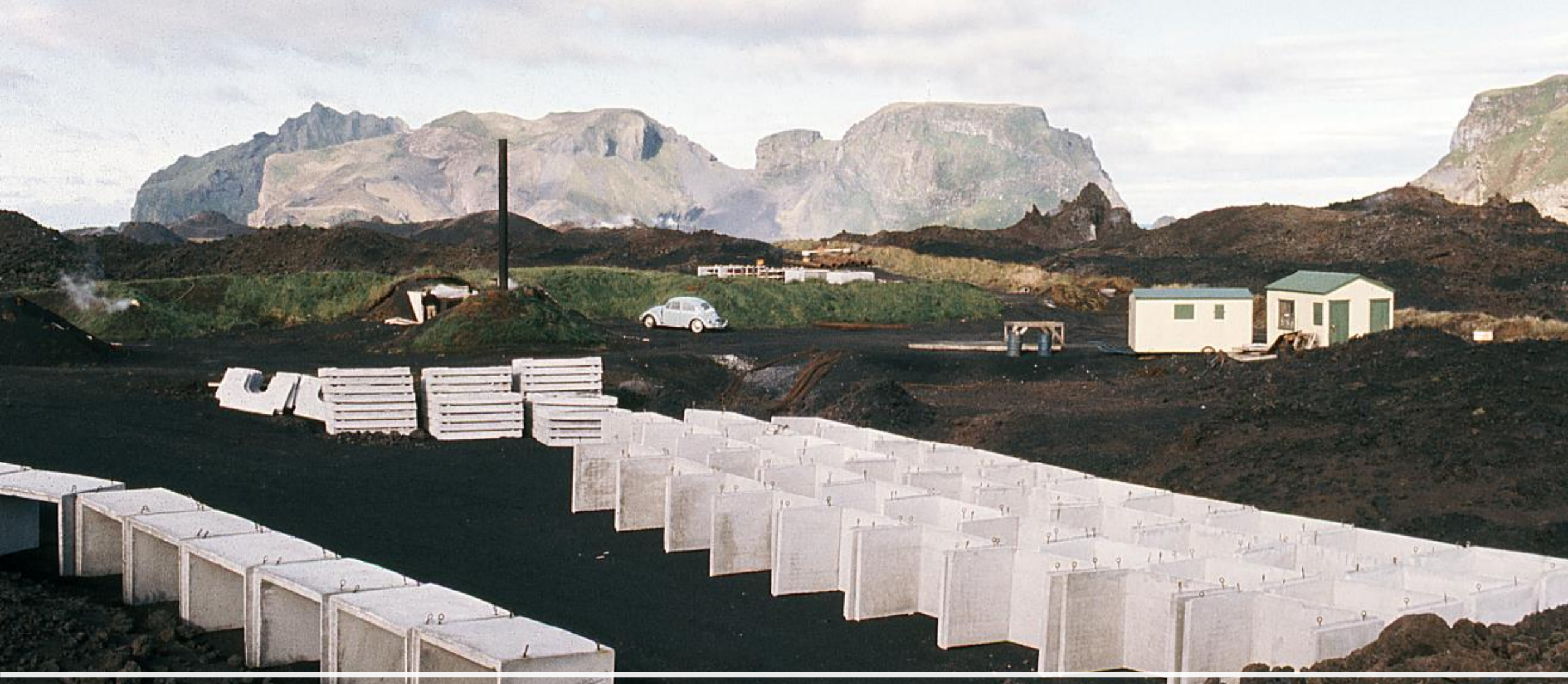
Concrete Cave cover over Heat Exchanger bundles
