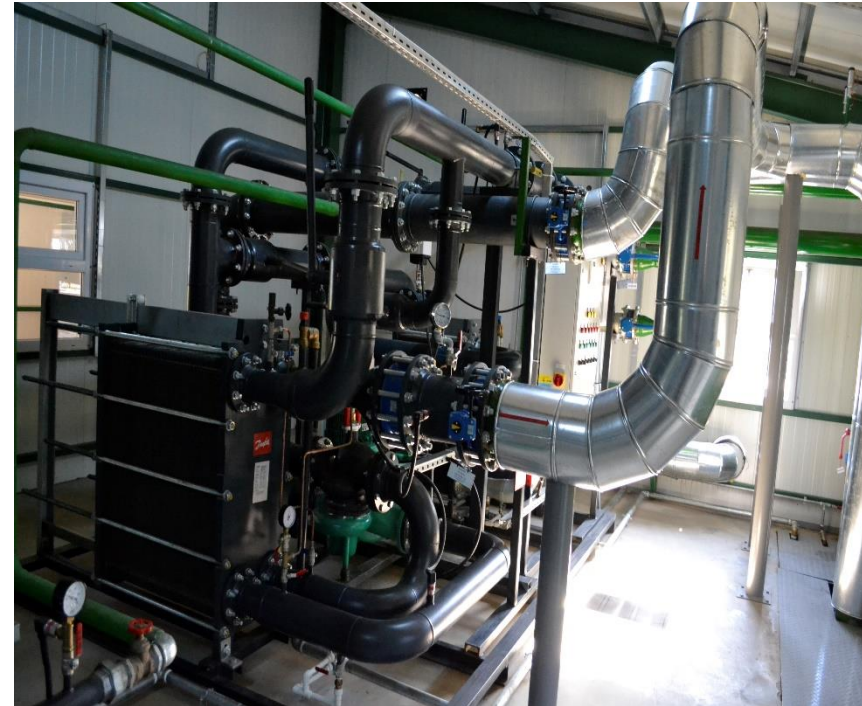
Exploitation unit of geothermal plant
