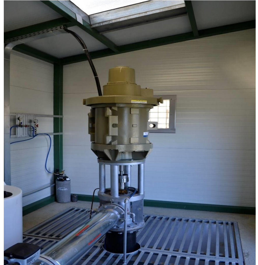
Line shaft pump in Balotesti well 2684 (25l/s)
