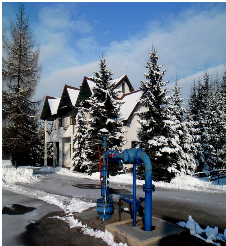
Podhale R.: first production well for geoDH in Poland (since 1992/93) Banska IG-1, MEERI PAS
